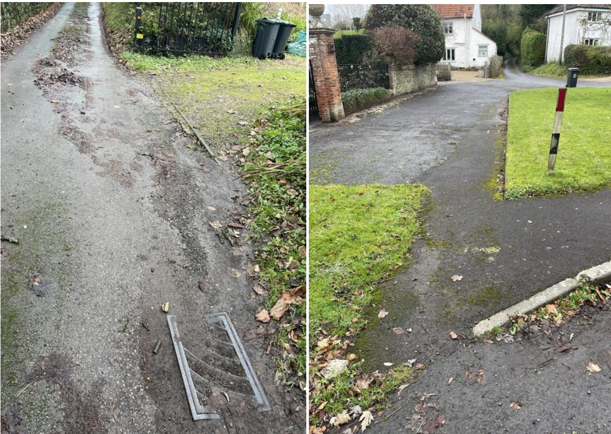
Soil, road debris and leaf litter blocking gully pots promoting flow onto roads and vulnerable low lying areas
